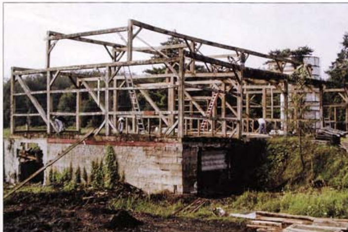
RIGHT: Beams from a 19th-century Wisconsin barn (above, during disassembly) became the great room's man-
